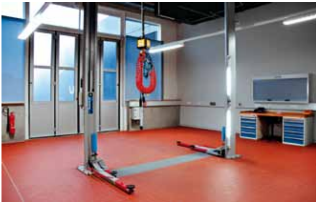
Secluded assembly halls with lifting platforms for your own technicians
