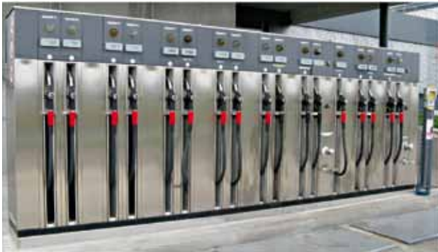
Refueling facilities with normal and certification fuel types
